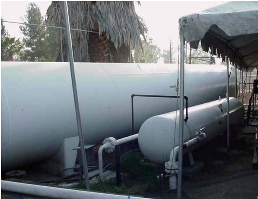
Compressed Air Storage
