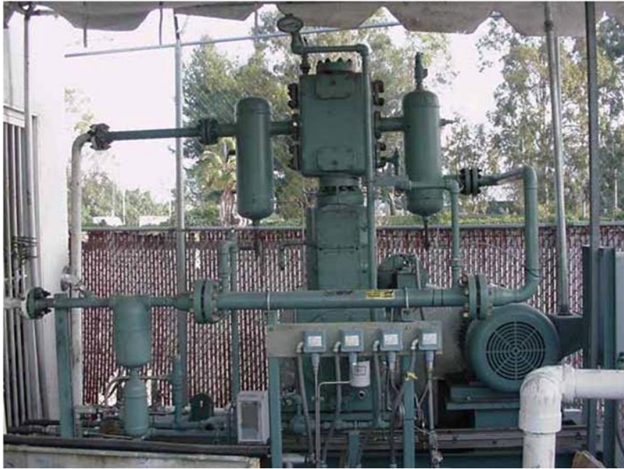
750 psig Boost Compressor
